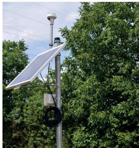
A weather station installed by the railway company in the danger zone, which, in combination with radar-based heavy rainfall forecasting, serves to assess the risk. These stations are to be set up in all danger zones, supplemented by radar-based systems that measure the intensity of heavy rainfall in the sub-areas more accurately than is offered by commercial weather data providers or the German Weather Service (DWD). Photo: sig Media GmbH
