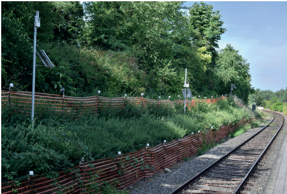
Two measuring chains provide data on the movement of the retaining wall (lower chain) and on landslides in the upper section. The left section is steeper, but has a rocky subsoil and is therefore not at risk. Photo: sig Media GmbH
