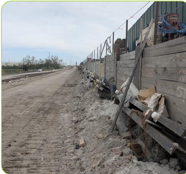
Senceive NanoMacros Triaxial Tilt Sensors deployed along a section of rail SoE
